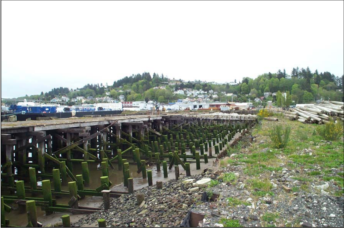
Photograph 27 - Looking southeast at ripped and bulkheaded Pier 3. Note weedy vegetation and wooden piles stored on Pier 3.
