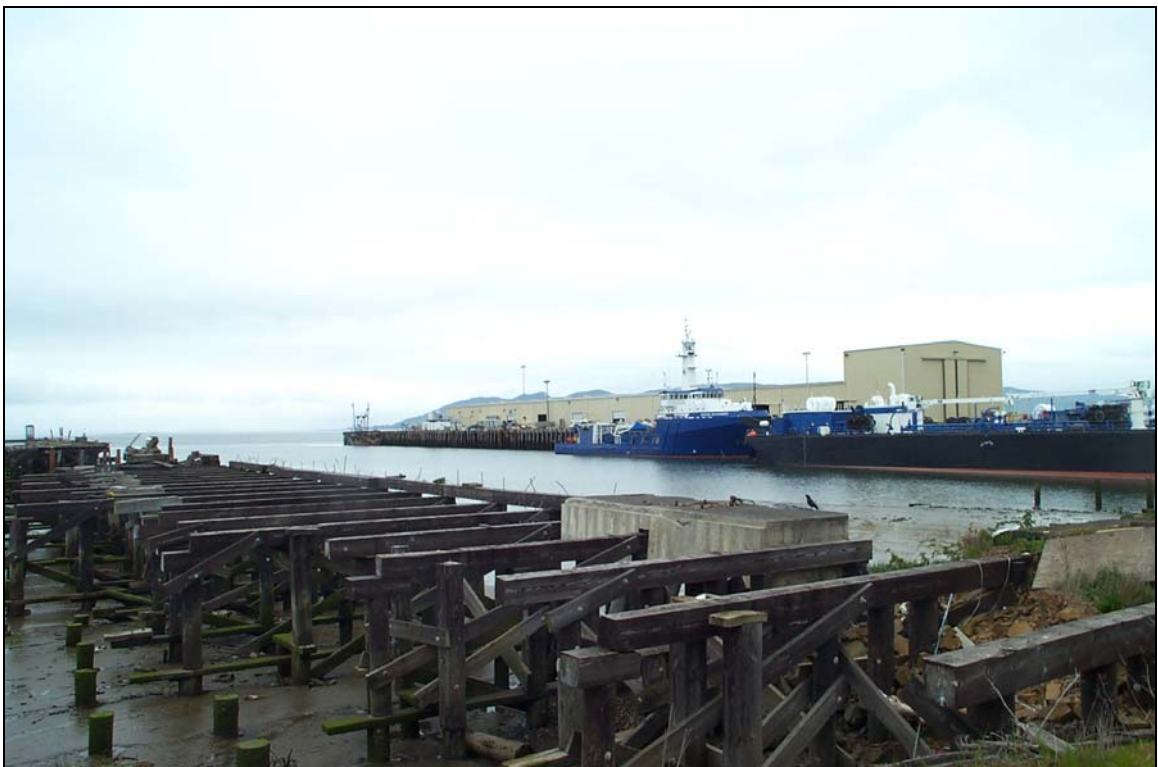
Photograph 26 - Looking north at dock ruins at Oregon Responder barge and tug from southwest corner of Slip 2 (Pier 3).
