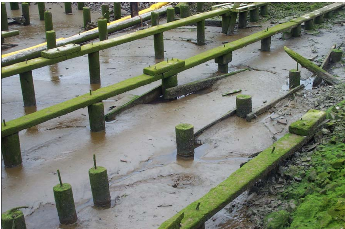
Photograph 24 - Closeup view of seep area. Note old wooden pilings along margin of Slip 2 and riprapped banks.
