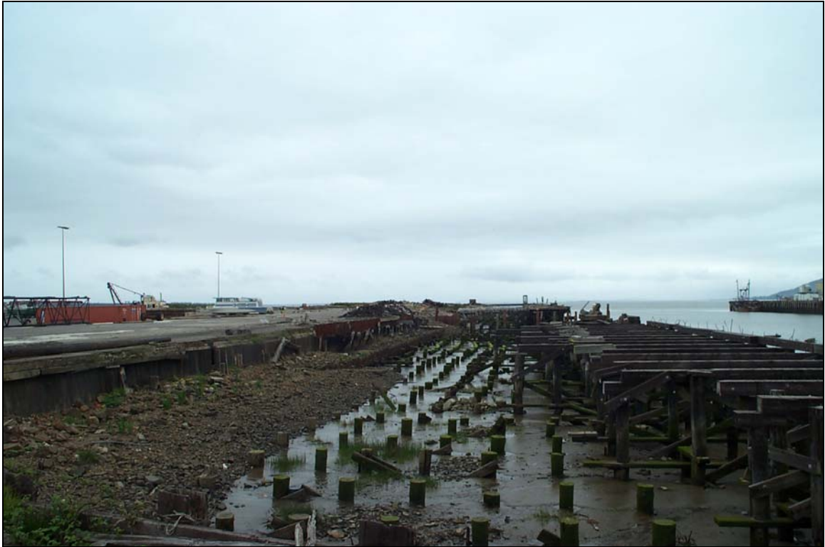
Photograph 25 - Looking northwest at dock ruins and pilings from southwest corner of Slip 2 (Pier 3 at left).
